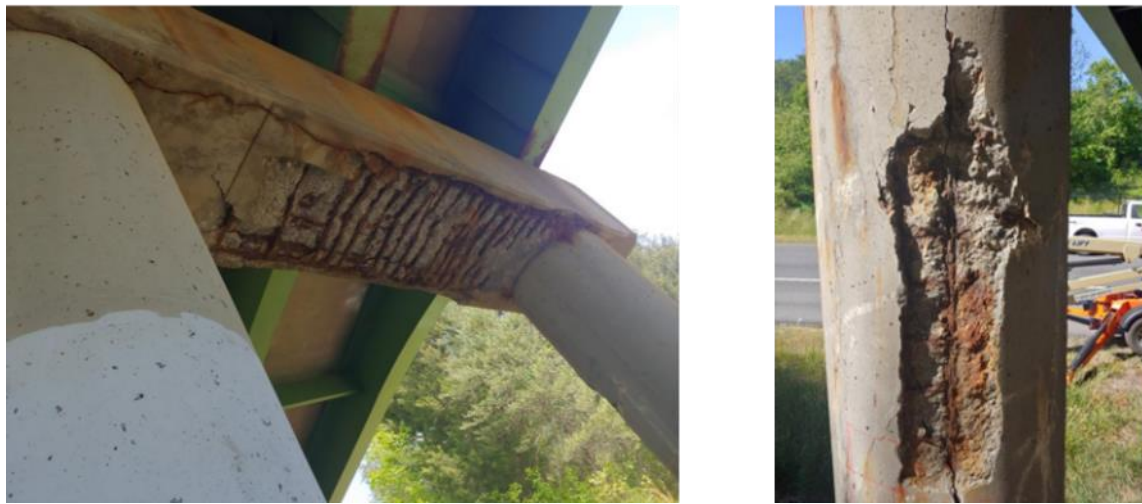
Figure 3. Corrosion on Pier 1 of the Route 605 Bridge
